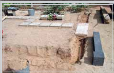
Hauapiirete paigaldus vundamendile. Установка оград на фундамент. Tombfence installation on the foundation.
